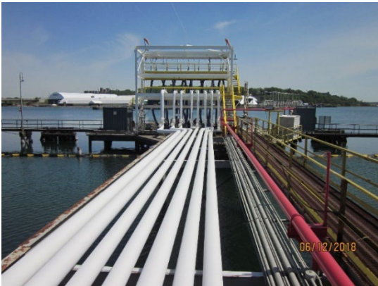
Old petroleum piping run, note location of pipes in relation to yellow railing to the right.
