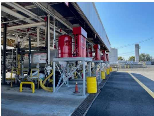
An example of an adaptation that elevated the fire suppression system above a level of concern.
