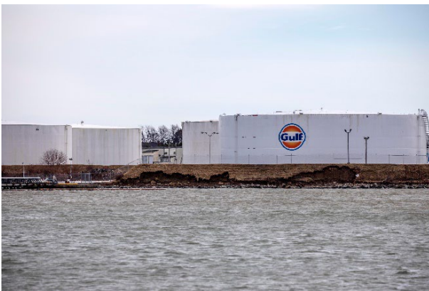
Erosion of tank containment wall from storm.
