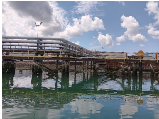
Petroleum piping run elevated as an adaptation for climate change. The old piping run was at the elevation of the middle yellow railing in this picture.
